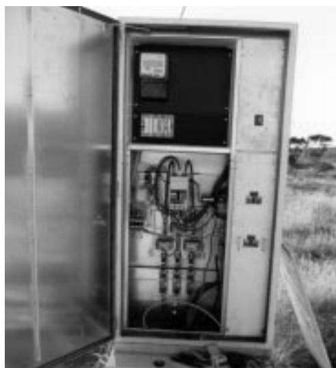
An electrician was tragically electrocuted whilst working in this switchboard
