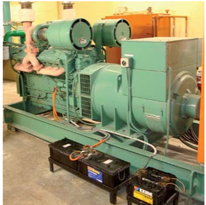
A typical diesel generator which may be suitable
