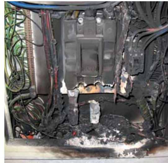
Use of the incorrectly connected meter destroyed this switchboard
