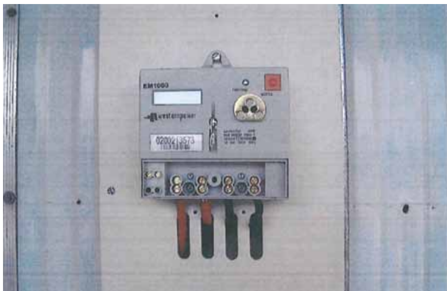
The transposed active and neutral conductors at the kwh meter. It should be connected red, black, black, red
