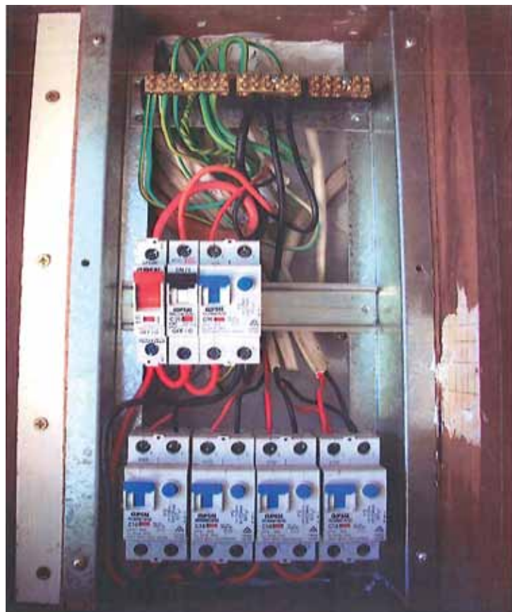
The main switchboard with the DIN rail kit frame not earthed.
