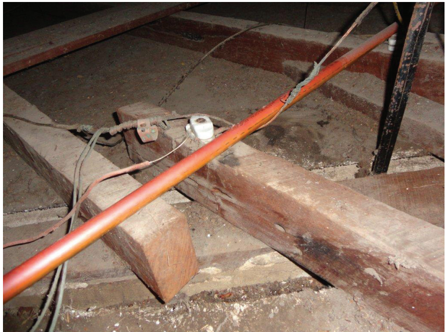
Picture depicts unsafe wiring near copper gas pipe
