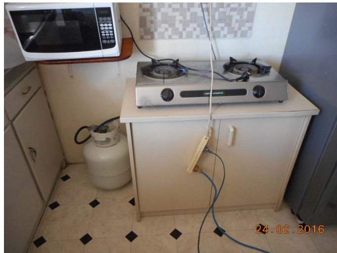
Wok type burner connected to an LP Gas cylinder inside
