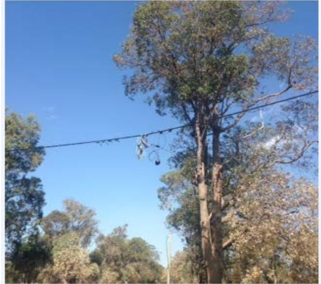
Loose wiring after the wooden pole it was attached to was destroyed by fire
