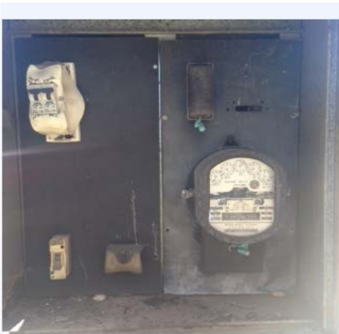
Melted switchboard attributed to the intense temperatures generated by the fire
