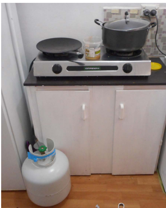
Wok type burner connected to an LP Gas cylinder inside
