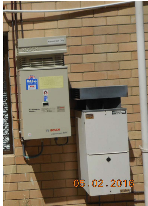
Installation of HWS on left is non-compliant also making the existing HWS on right non-compliant
