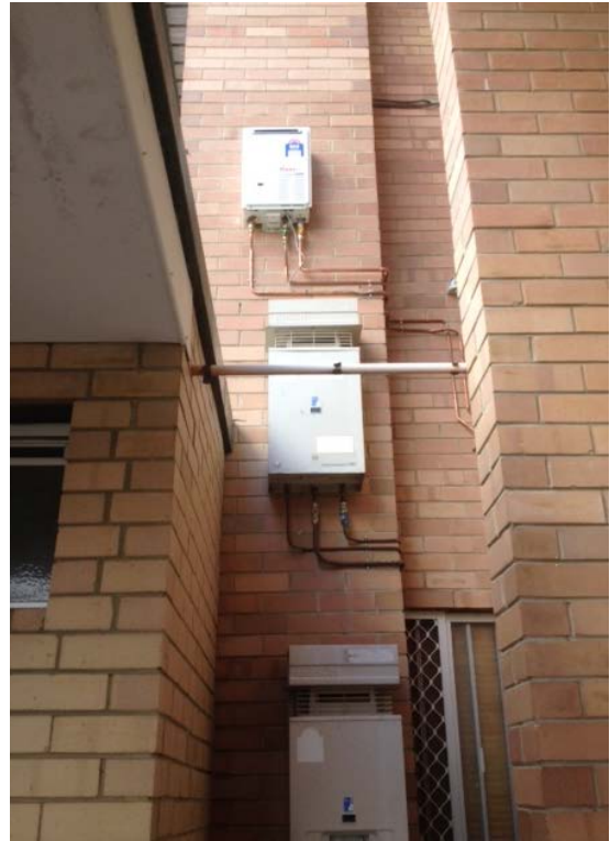
Non-compliant water heater installations
