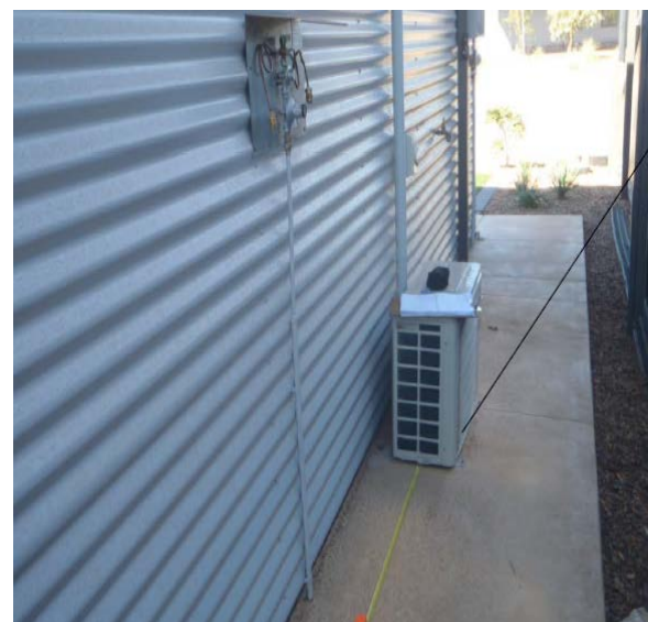
Air-conditioner condensing unit installed in a restricted zone near gas cylinder pigtails and pipe work
