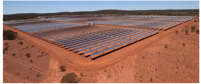
Solar installation at DeGrussa mine
