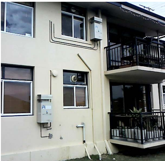
Non-compliant water heater installations
