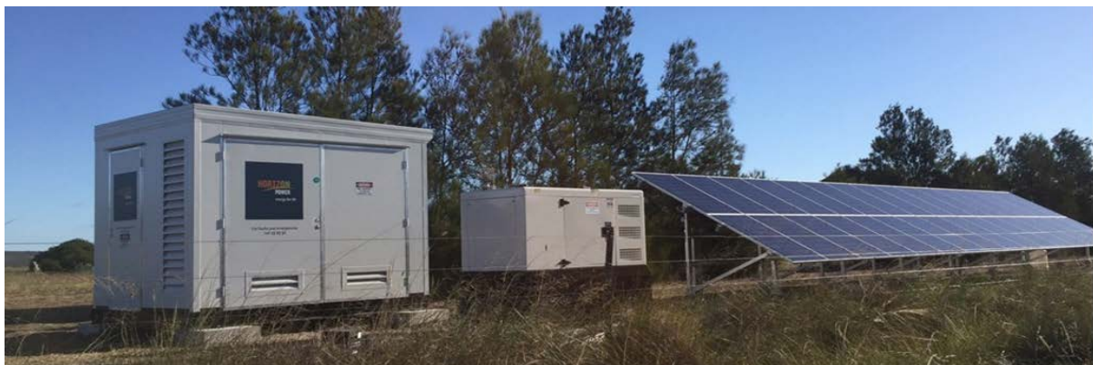
Off-the-grid power solution comprising photovoltaic arrays and battery storage
