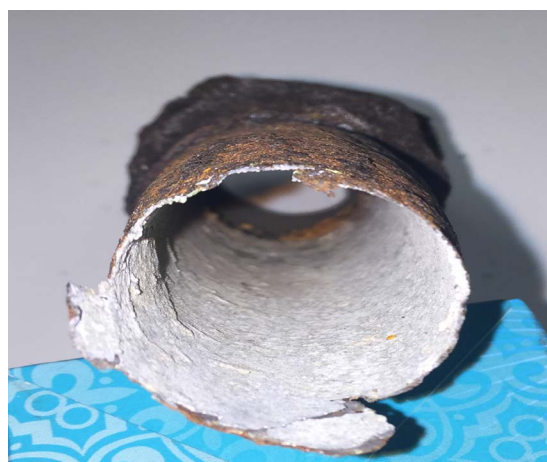
Rusted galvanised wrought iron pipe
