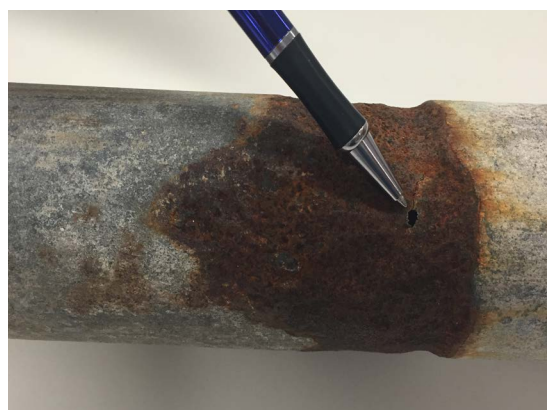
Hole in galvanised wrought iron pipe
