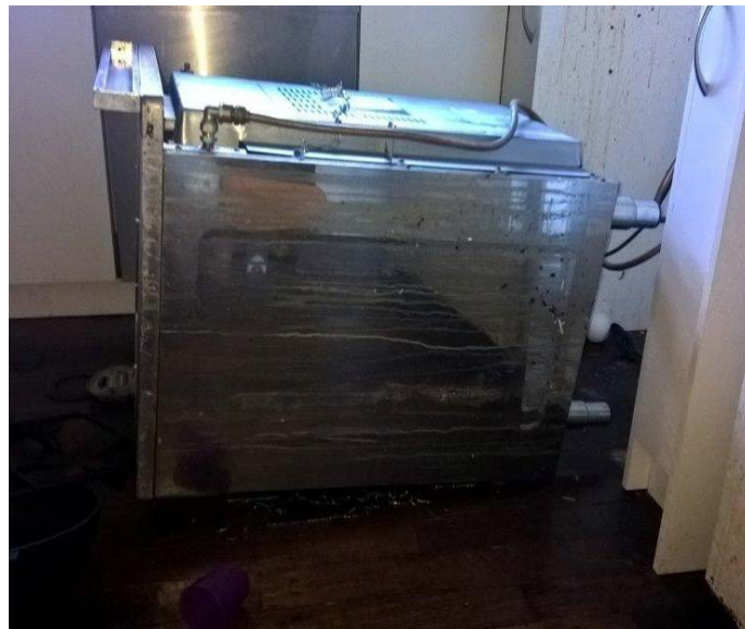
Result of non-compliant installation
