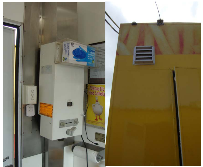
Gas water heater with a modified flue
