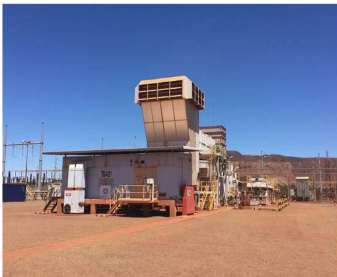
The gas turbine (Alinta Power) installed at Newman
