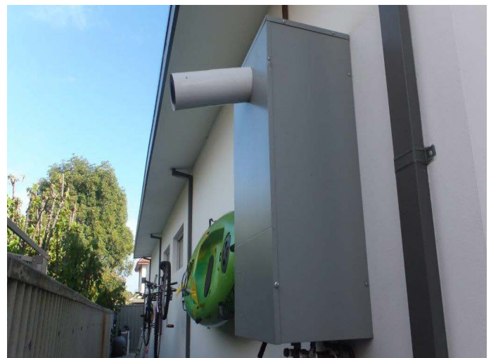
Non-compliant Combi-boiler installation
