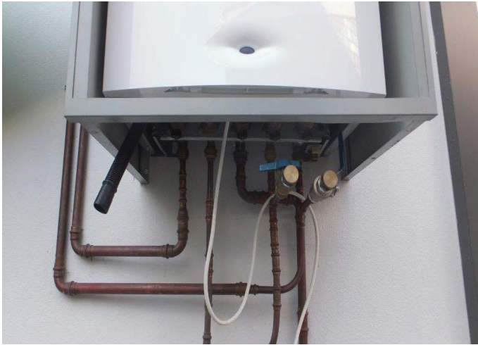
Non-compliant combi-boiler installation
