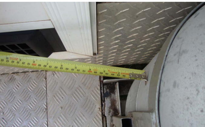
LP Gas cylinders installed too close to the air vent
