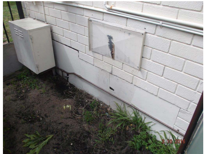
Natural gas meter box and pipe
