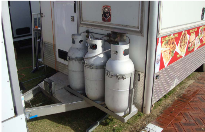
LP Gas cylinders installed too close to the entrance
