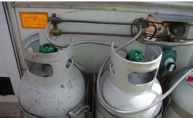
No insulating strips were installed between the cylinders and their clamping bands
