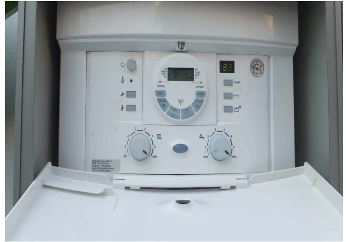
Panel of the combi-boiler
