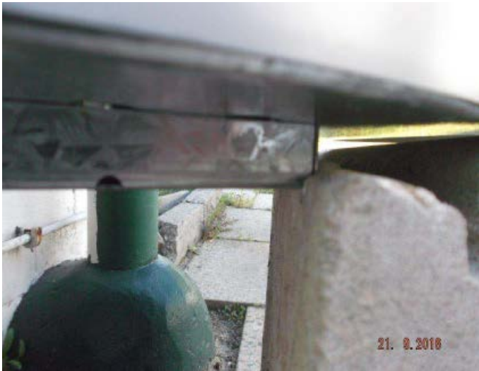
Base of the hot water system balancing on the paver
