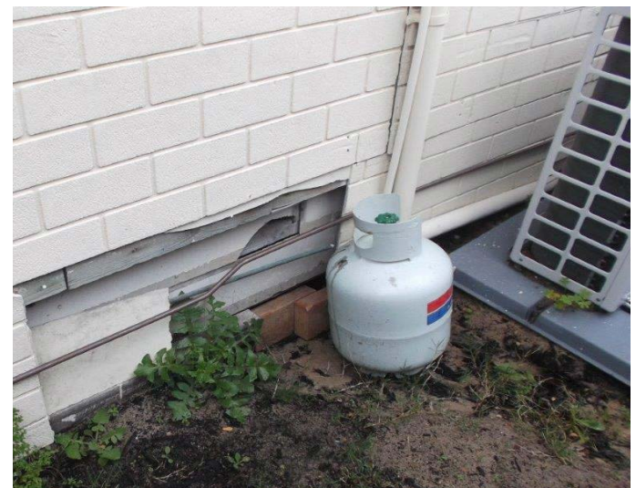
LP Gas installation
