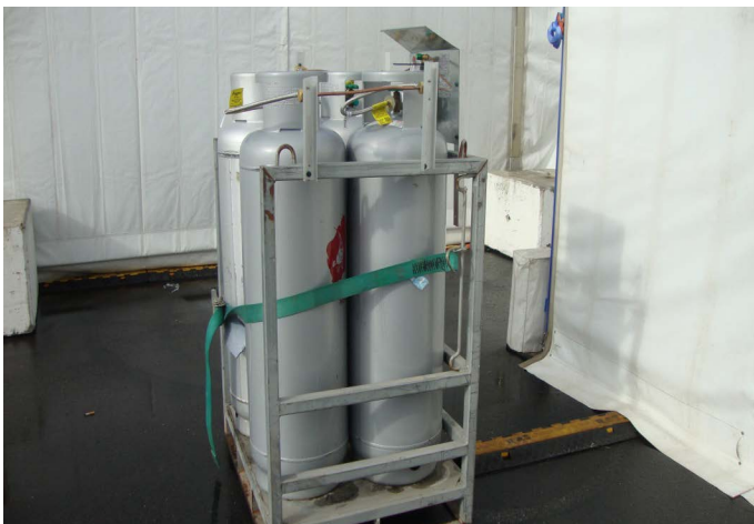
4 x 45Kg LP Gas cylinders secured in a cage
