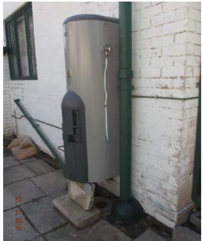
Hot water system propped up on pavers
