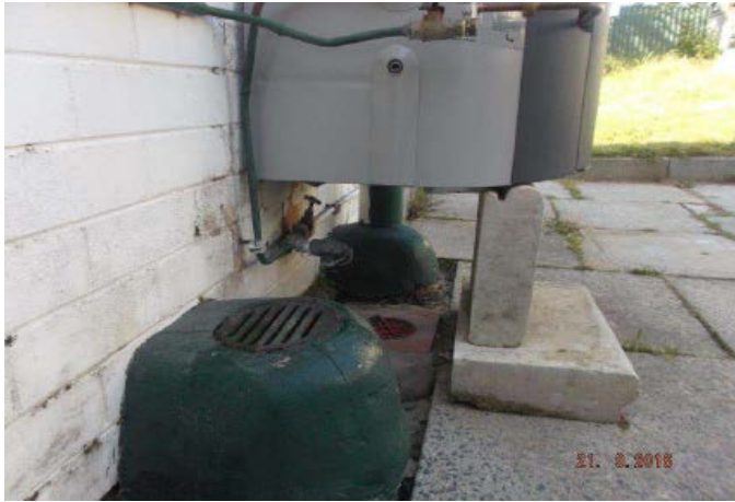
Hot water system installed above a tap
