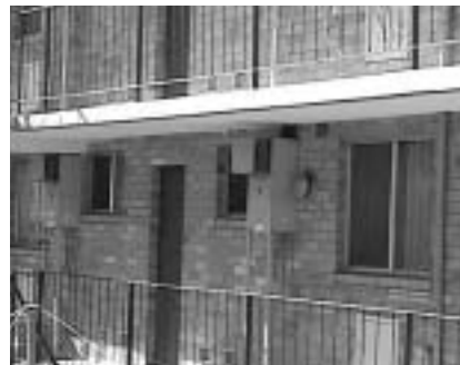
Typical water heater installation that will require an exemption
